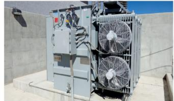
SUBSTATION TRANSFORMERS for Indoor & Outdoor operation
